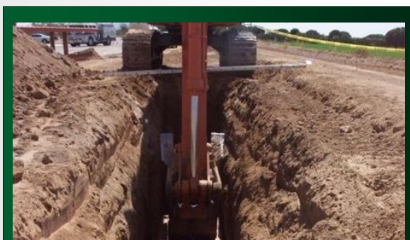
ACOG worked on the administration of an ARC grant a to construct sewer lines along Highway 5
